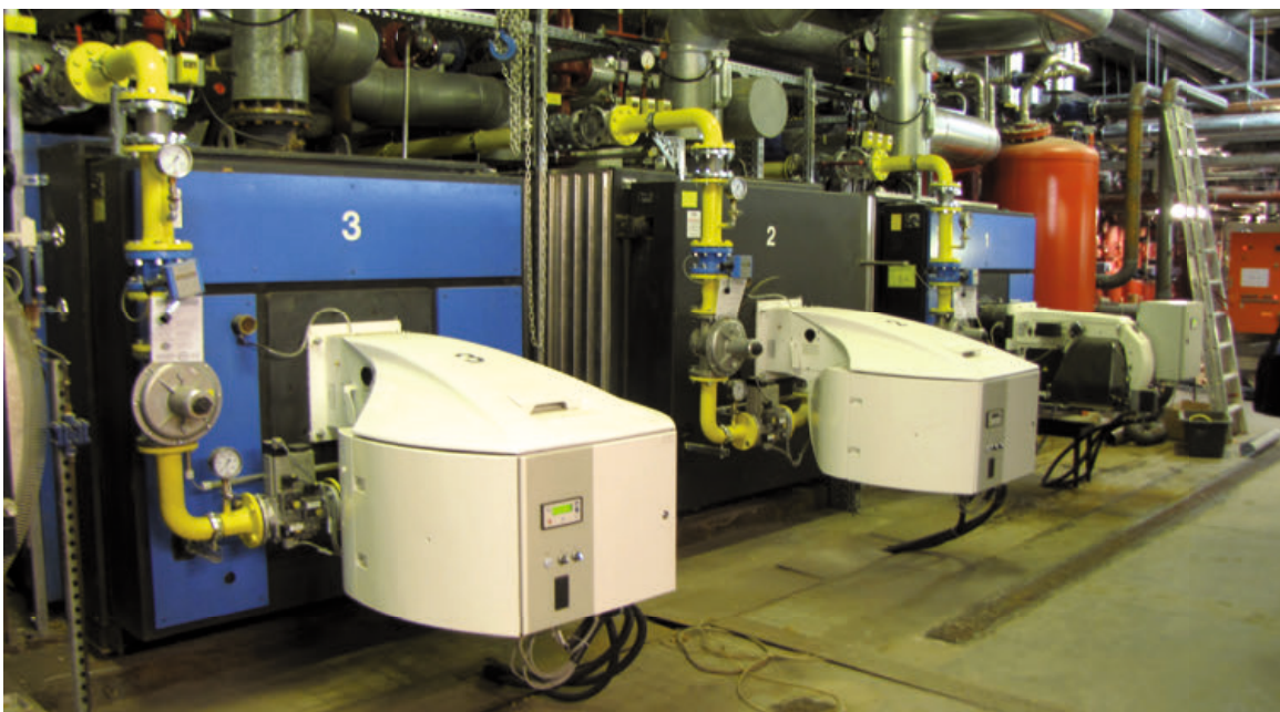
Fig. 92: 167 tonnes of hot steam per hour can be supplied by the boiler for the propulsion of the steam turbine and supporting the district heating supply
