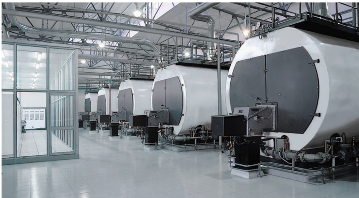
Fig. 91: Five gas-operated high-pressure steam generators, each of which produce 16 tonnes of steam per hour at an operating pressure of 10 bars
