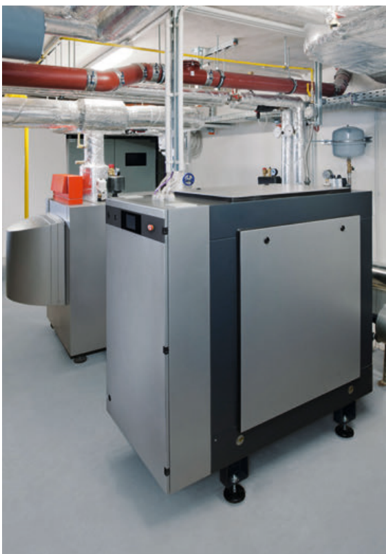
Fig. 47: CHP plant in combination with a peak load boiler for supplying an apartment building.
